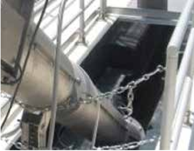
Insulation against low temperature in the compaction and transport zone
